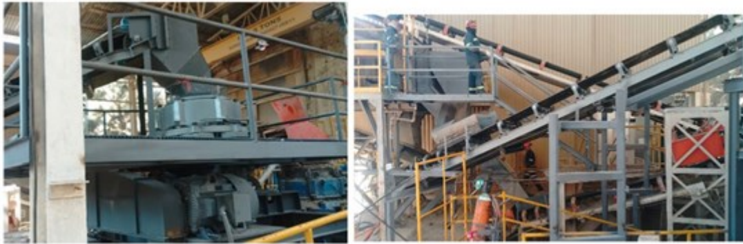
Figure 2: New cone crusher and conveyor
